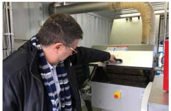
The Salsnes Filter system producing a highly-concentrated cellulosic primary sludge.
