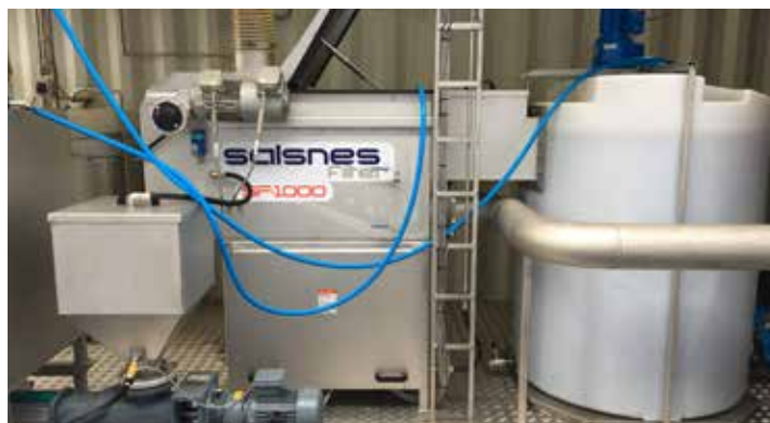
A SF 1000 Salsnes Filter installed at the Carbonera WRRF as part of a SMART-Plant demonstration project.
